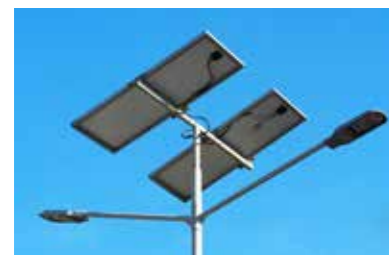
路灯 street lamp
